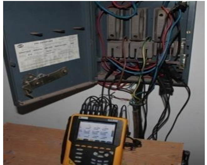
Fig. 6. Chauvin Arnoux CA 8335 power quality analyzer (PQA) used for data measurement
