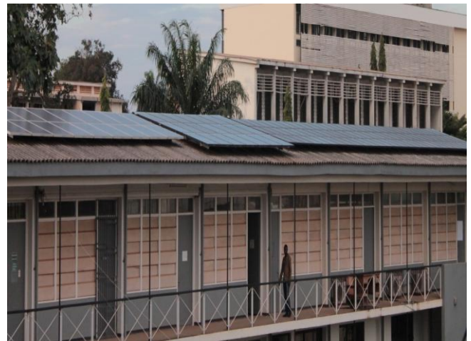
Fig. 3. 12 kWp solar panels at the Lecture Theatre (LT) Block
