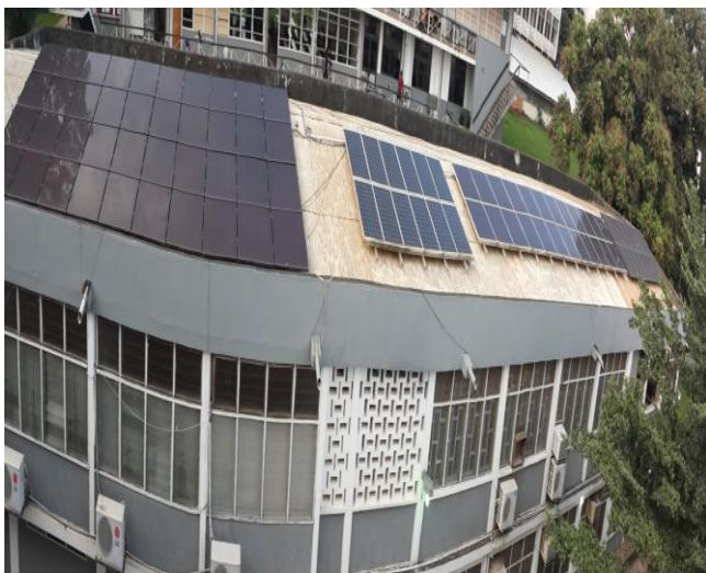
Fig. 2. 12 kWp solar panels at the Engineering Professorial Block (PB)
